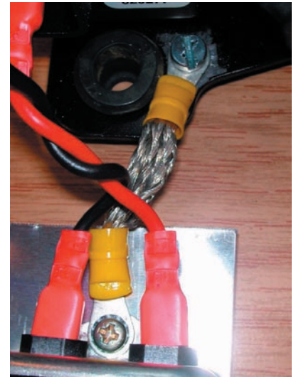
Ground connection between the compressor and the filters
