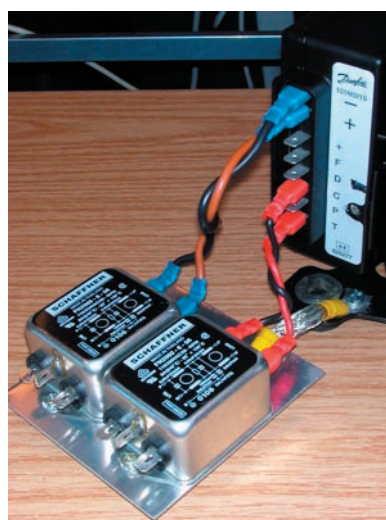
The base plate of the filters is connected to the compressor base plate by using a grounding point
