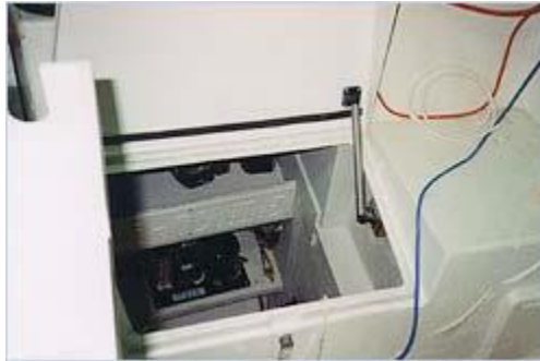
Shows Nova Kool LT200 installed in ventilated lazarette.
