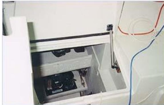
Shows Nova Kool LT200 installed in ventilated lazarette.
